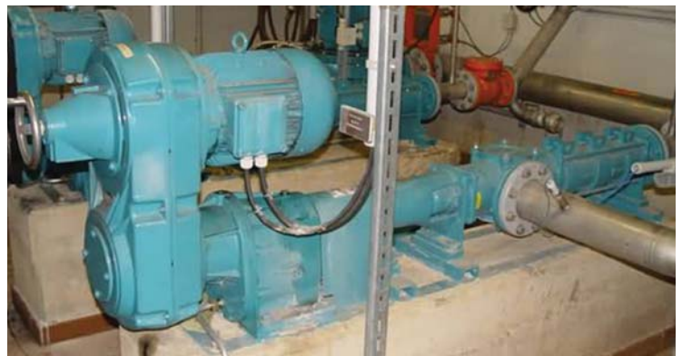
Time control and highly efficient direct-drive motors (EFF1) have replaced these belt-driven SEP Series primary sludge pumps.
