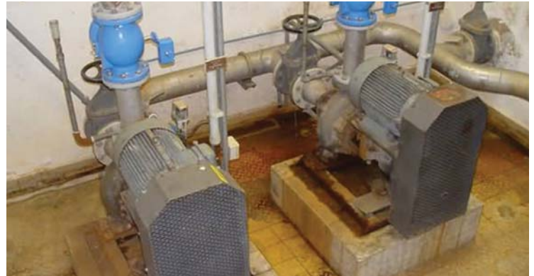
Allweiler’s optimization recommendations made it possible to eliminate these two centrifugal pumps, saving the plant energy and maintenance costs.
