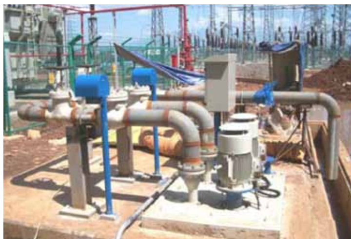
Installed sump pump package
